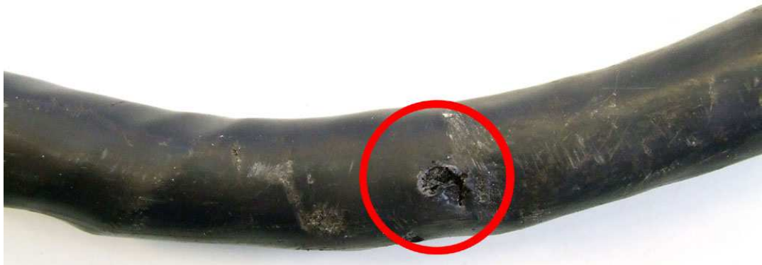
Figure 19: the burn mark on the surface of the faulty cable
