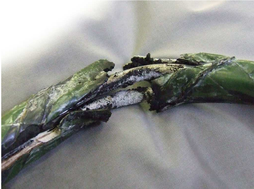
Figure 20: the wires of the opened cable with the burnt insulation
